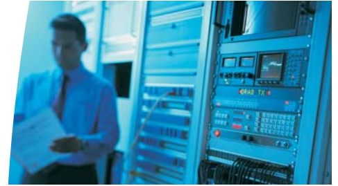
Servers, data storage and network equipment.
